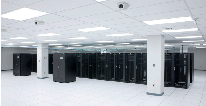
Each side of Temple's data center has space for six rows of cabinets
