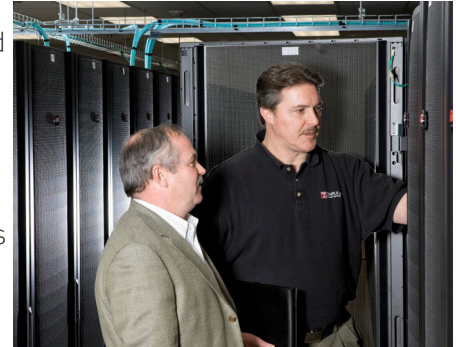
Dave Hollie of ITS and Mike Taylor of Temple examine the new data center infrastructure
