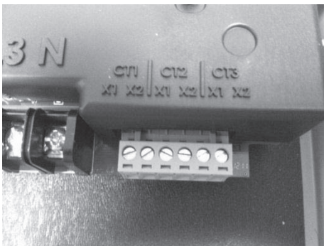
CT Terminal Block in Place
